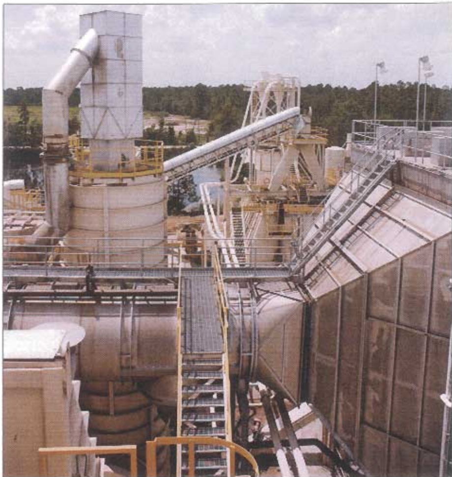
Georgia-based Teaford supplied wood fiber burners and two energy systems.
